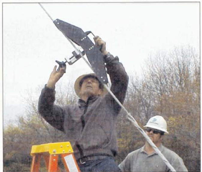
The PIAB RTM 20 D allows crews to determine the tension of a guy before they move it.
