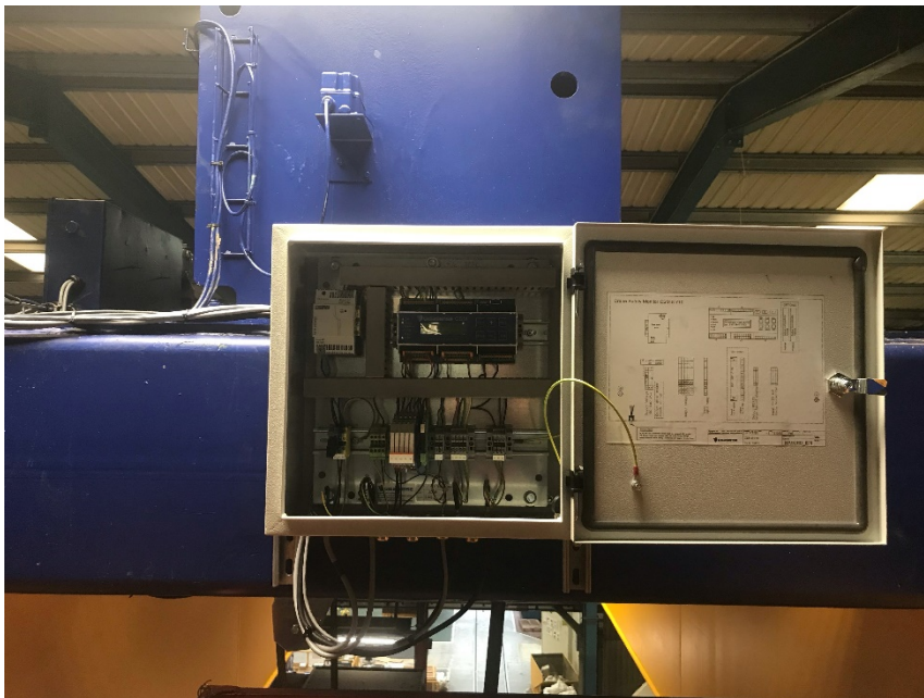
Picture: Crane Safety Monitor – CSM, installation
